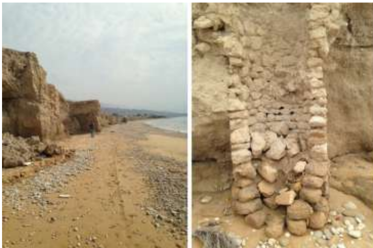
Figure 28: Photographs of the coastal erosion at the base of Siraf's old city walls (Group 3 transects).
